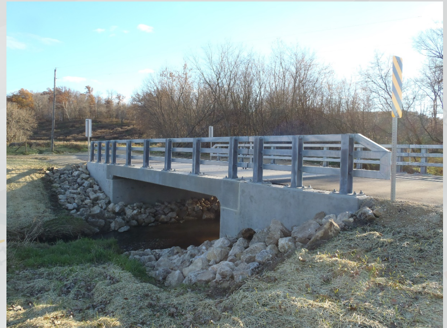
Single Span Bridge with Type M Railing Wings Parallel to the Road
