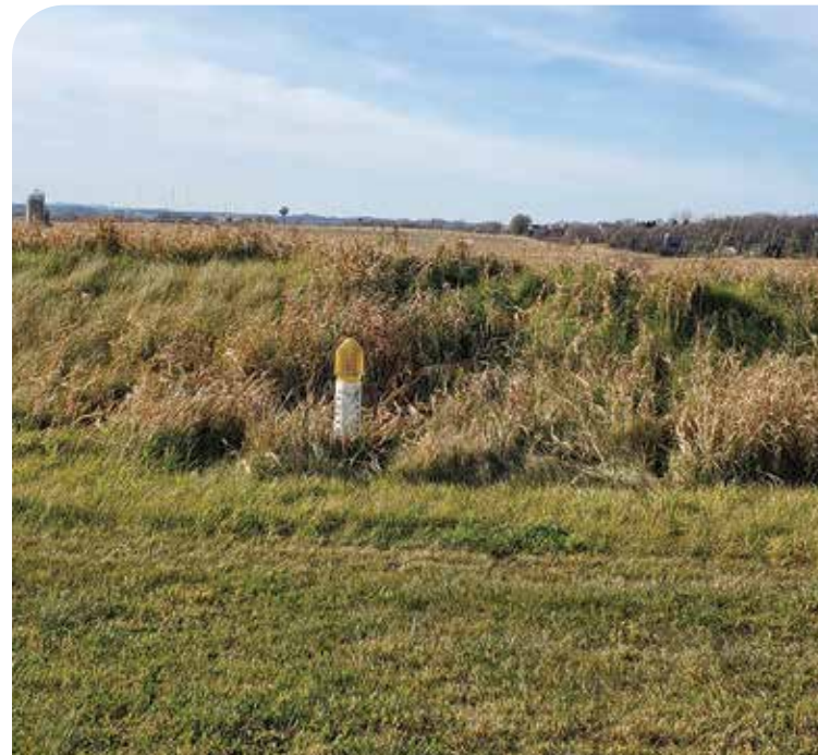
A water and sediment control structure constructed by Dane County LWRD staff in 2015.
