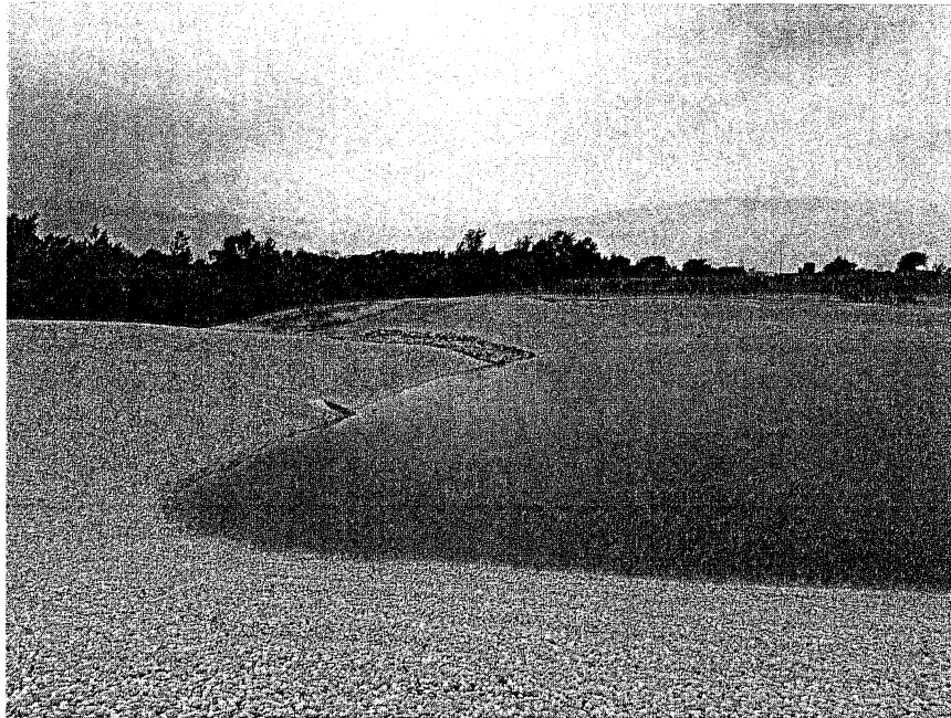
Photo 3: South portion of completed pond. Southern concrete pipe inlet and spillway (Looking West) (06/22/15)
