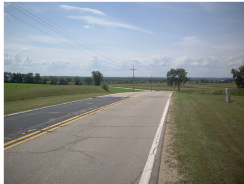
Facing south on CTH F. Poor pavement condition, sharp horizontal curve, poor site distance.
